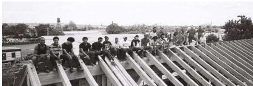
Trainees and Challenge Program staff on top of the erected timber frame.
